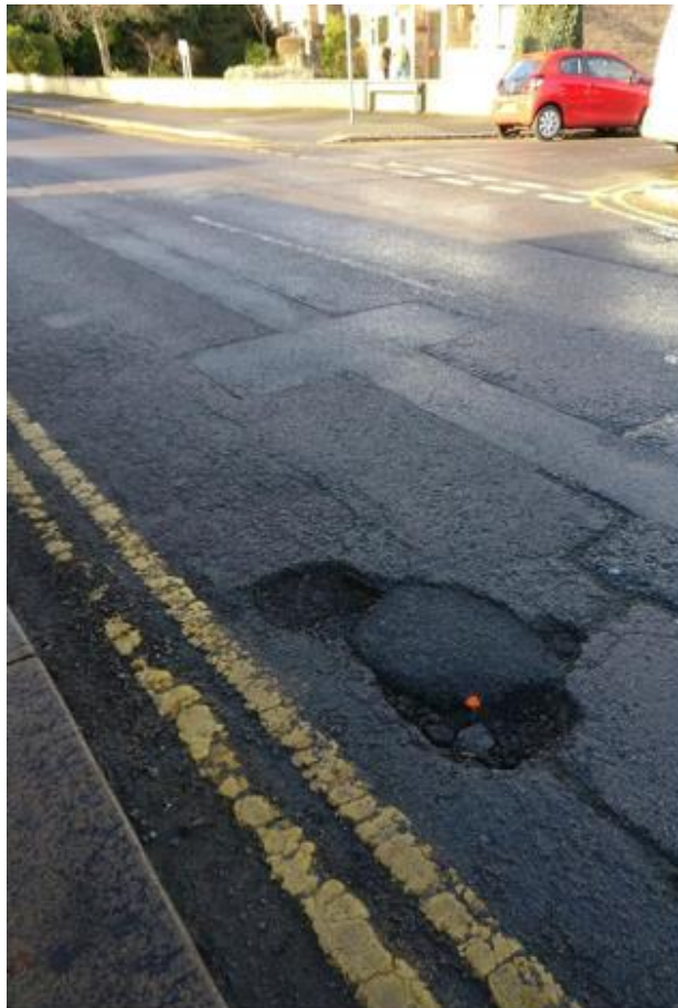
Before - three defects treated as one single defect
